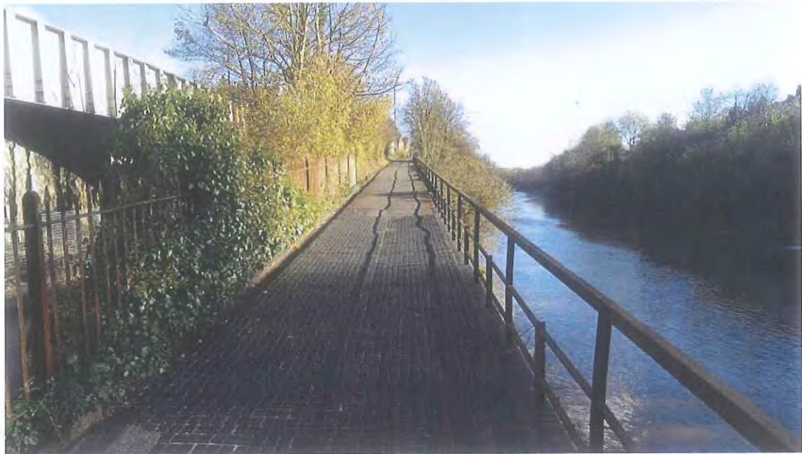
Chocolate Path ramp to Cumberland Road – tarmac patching can be seen further along path.
